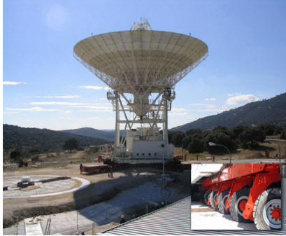
Giant Deep Space Network antenna in Madrid is moved using four 12-axle, 24-wheel crawlers.
